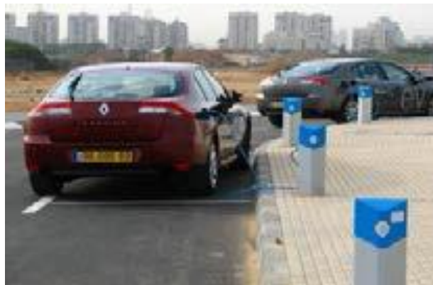
Figure 29: Off-street and robust charger at commercial and office area
