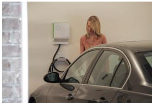
Figure 28: Domestic charger at residential area
