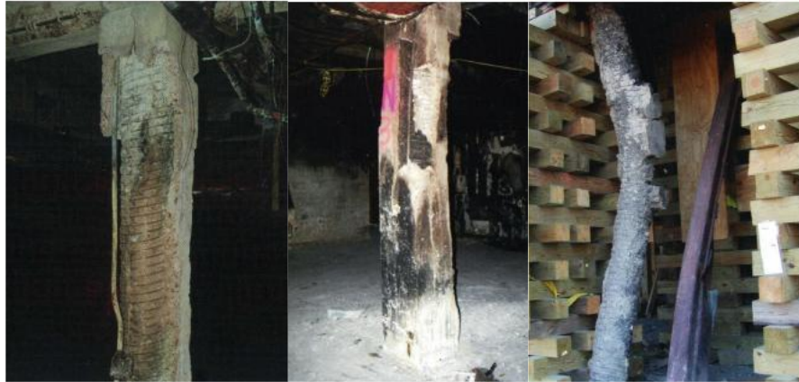
Fig.1. 2Spalling-damaged heat-exposed columns (Pentagon, Washington, USA, 2001).
