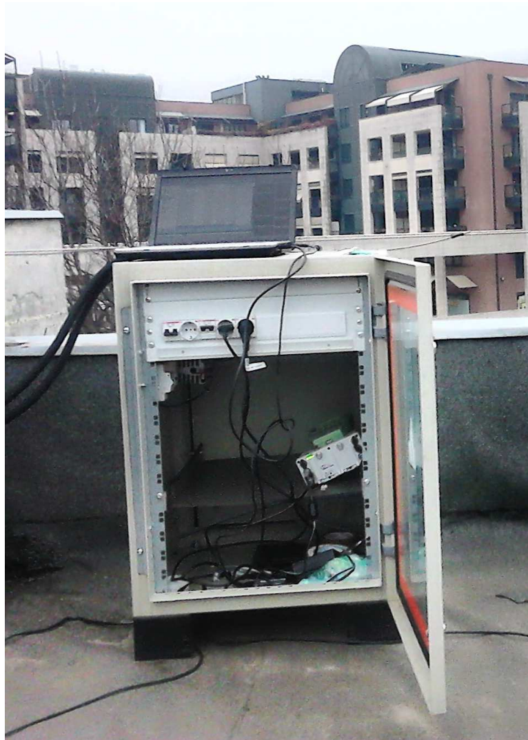
Figure 2.9 – The rack used to power the devices using during the test
