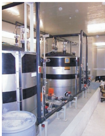
(a) Tanks for CESI plant
