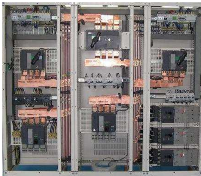
Figure 1.16 The interior of a switchgear
