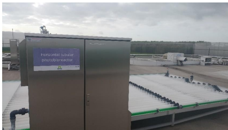
FIGURE 2.3.7: HORIZONTAL TUBULAR PBR (WAGENINGEN UNIVERSITY, ALGAEPARC PILOT FACILITY) (ALGAEPARC, 2018)
