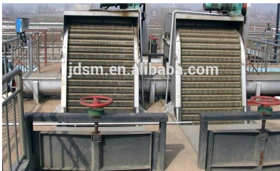
FIGURE 2.3.13: MECHANICAL TRASH RACK RAKED BAR COARSE SCREEN (ALIBABA, MECHANICAL TRASH RACK RAKED BAR COARSE SCREEN, 2018)
