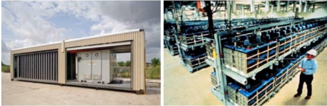
Figure 15 Lead-Acid Battery Storage system; left: Xtreme Power 1 MW - 1 MWh; right: Electric Power Research Institute of California 10 MW – 40 MWh
