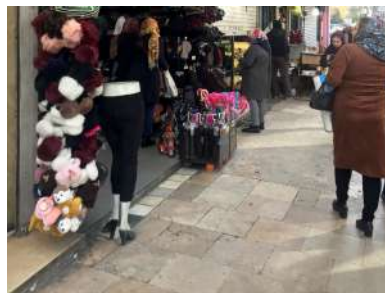
Figure 123: Tiles in a good condition in a leading street to Tajrish Square (Self Elaboration)
