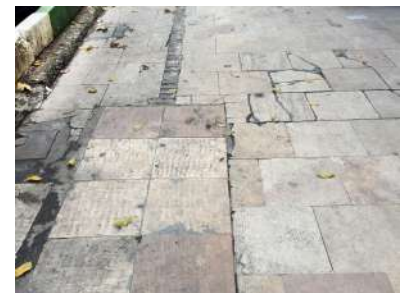
Figure 124: Tiles in a bad condition in a leading street to Tajrish Square (Self Elaboration)
