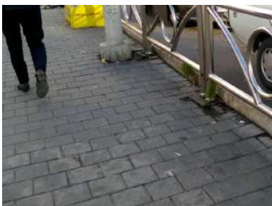
Figure 122: Tiles in a good condition around Tajrish Square (Self Elaboration)
