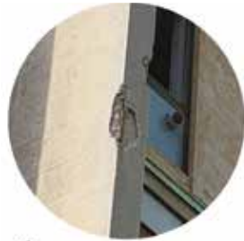
4 Fig. 02.93 Exposed rebars
