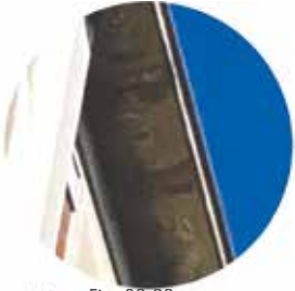
3 Fig. 02.92 Water leakage causes staining on roof eaves
