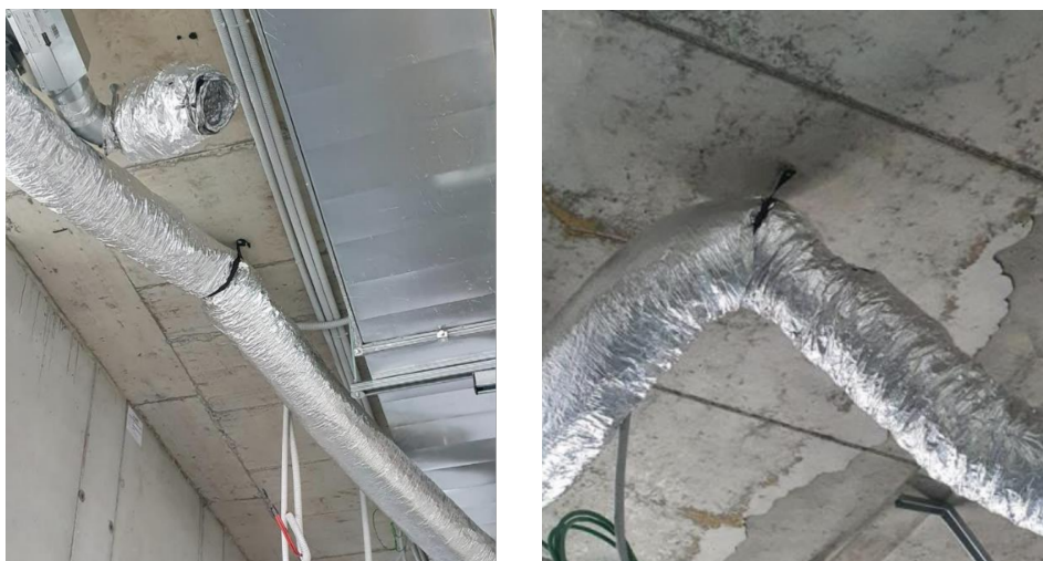
Figure 3.14: Air supply ducts constrictions
