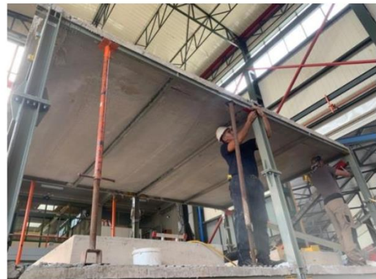
b. Replacement of DRBeS
