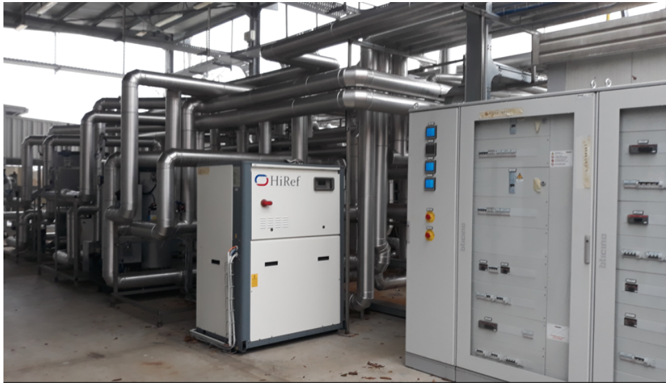
Figure 3: A view of the RSE Test Facility (image taken from [24]).
