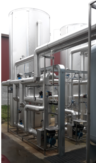
Figure 1.11: Photo of the Test Facility thermal storages.
