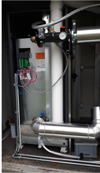
Figure 1.4: Photo of the gas boiler implemented in the RSE Test Facility.
