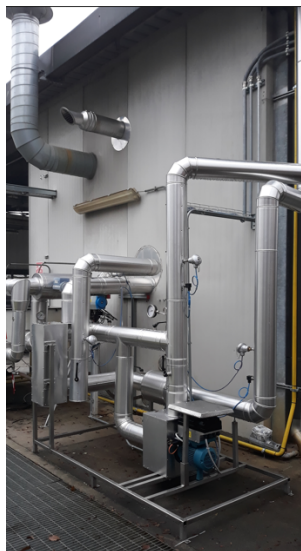
Figure 1.8: CHP system of the RSE Test Facility.
