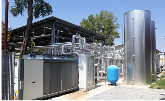
Figure 1.18: Chiller of the RSE Test Facility.
