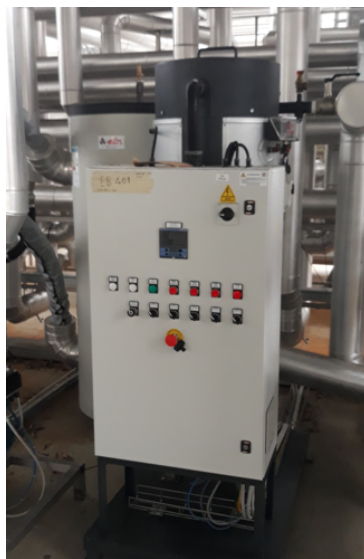
Figure 1.6: Photo of the electric boiler used in the RSE Test Facility.
