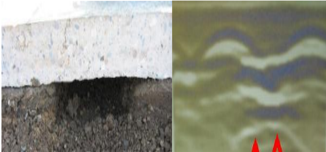
Figure 2.16: Void in concrete on the left and GPR image of void in concrete on the left
