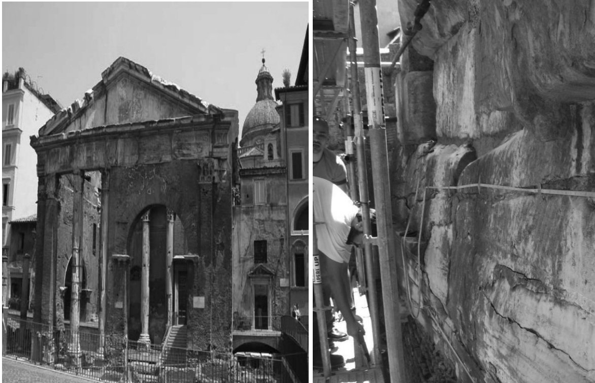
Figure 2.7: The archaeological site of Porticus Octaviae (left) and the poor state of conservation of marble of the Porticus Octaviae (right)
