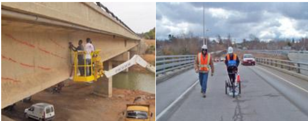
Figure 2.32: BridgeScan GPR assessing bridge deck, reinforced concrete (left) and road structure (right).
