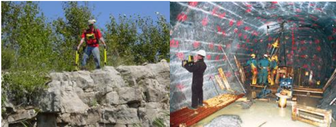
Figure 2.21: Rock Noggin GPR being used on hard rock and inside a tunnel.
