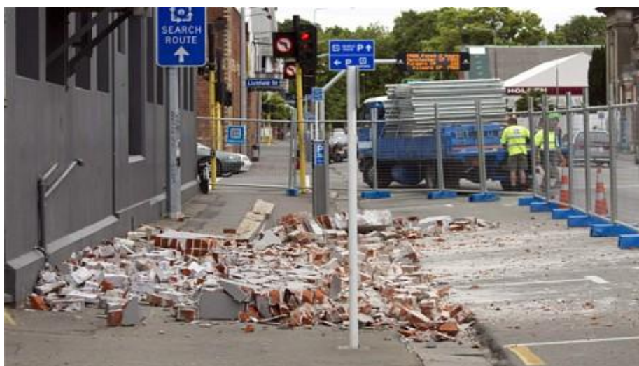
Figure 1-10: Collapse of non-structural masonry wall (Christchurch, 2011)
