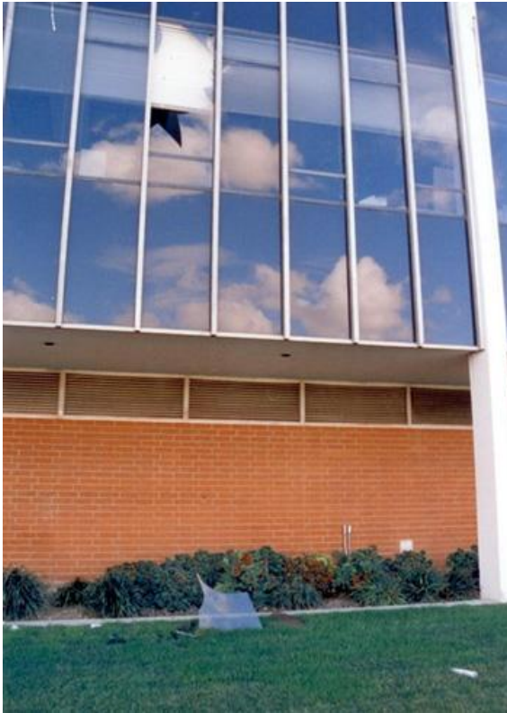
Figure 1-23: Glass shards fallen from a curtain wall frame. (Northridge, 1994)
