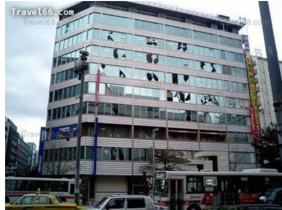
Figure 1-26: Damage and glass shards fallout from facade frame. (Fukuoka, 2005)
