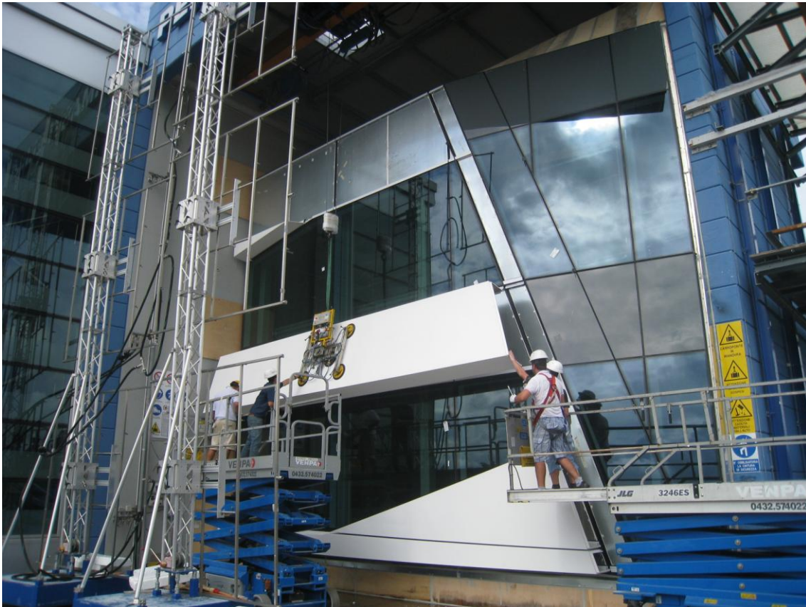
Figure 4-5: Outside view of the Permasteelisa mock-up performance test facility (Courtesy of Permasteelisa S.p.a.).
