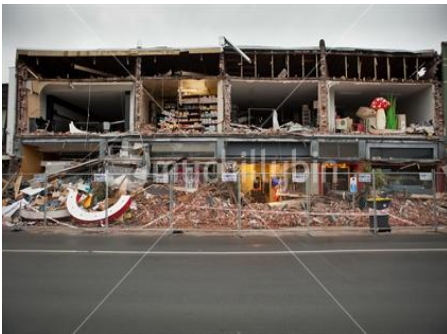
Figure 1-8: Damage to non-structural exterior masonry walls (Christchurch, 2011)
