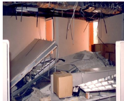
Figure 1-9: Damages to internal furnishing and ceilings collapse (Northridge, 1994)
