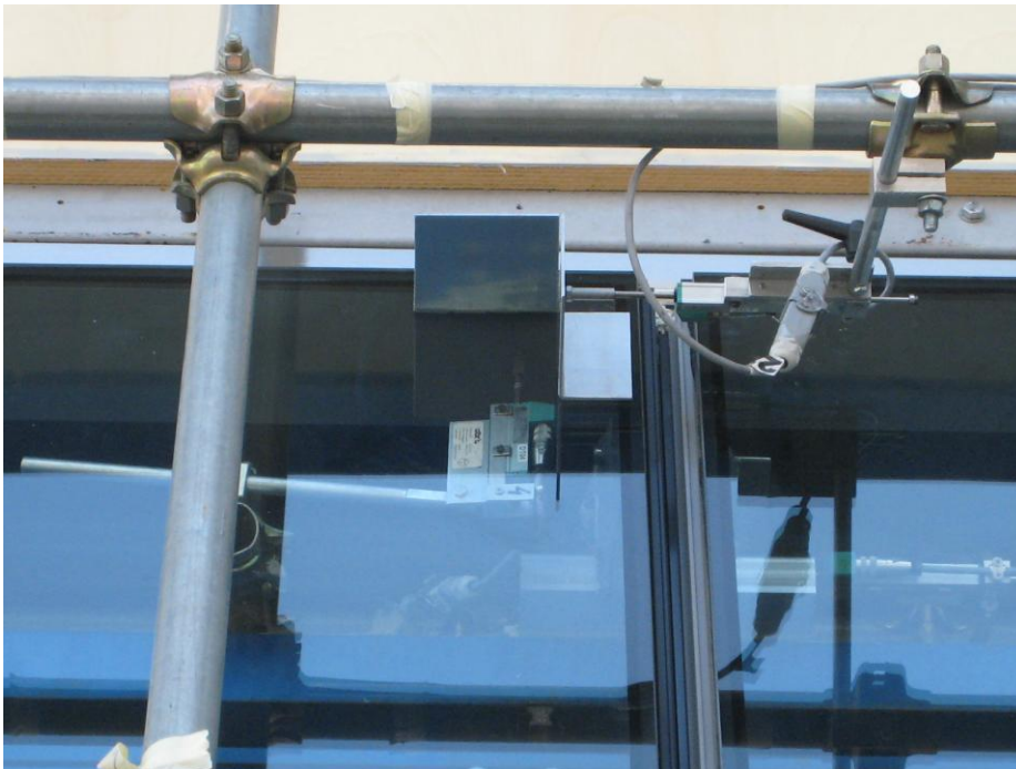
Figure 4-22: Detail of the DT-13 displacement transducer placement for the vertical movement recording at the upper corner of the glass (Courtesy of Permasteelisa S.p.a.).
