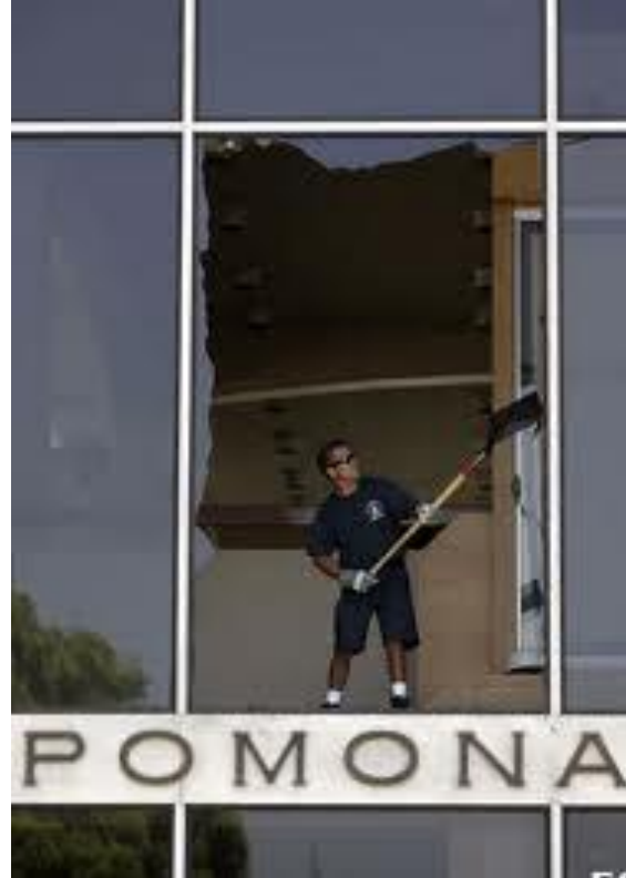
Figure 1-24: Maintenance operations after glass damage and fallout from the curtain wall frame. (Northridge, 1994)
