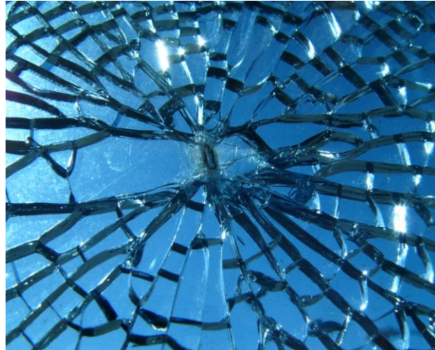
Figure 1-28: Typical example of fully-tempered (FT) glass breakage.
