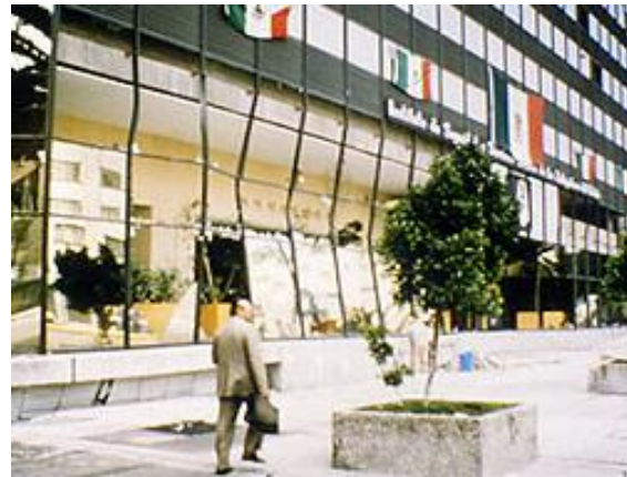
Figure 1-32: Aftermath of an earthquake to a stick curtain walling system. (Mexico City, 1985)
