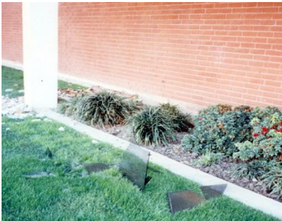
Figure 1-31: Glass shards fallout from a curtain wall. (Northridge, 1994)
