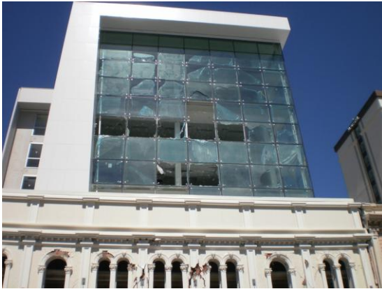
Figure 1-25: Aftermath of an earthquake on a structural glazing curtain walling system. (Christchurch, 2011)
