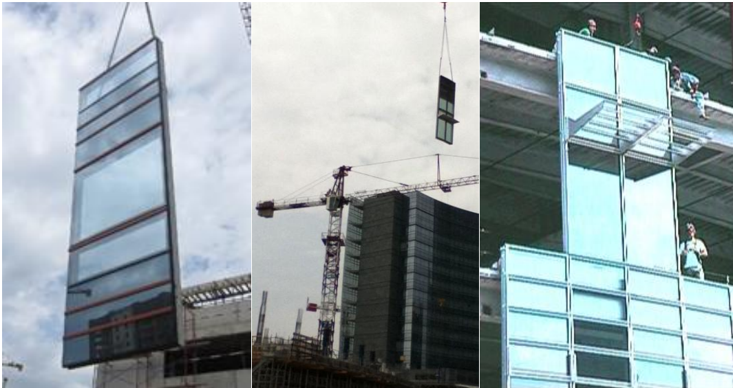
Figures 1-15 /1-16 /1-17: Several moments during the installation phase of a unitized curtain walling system.
