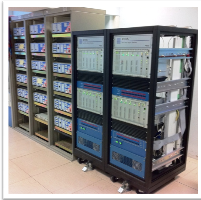
Fig. 4.2-1. The RTDS (on the right side), with the amplifiers bank (on the left side), installed in the Enel Distribuzione Test Center (Milan, Italy)
