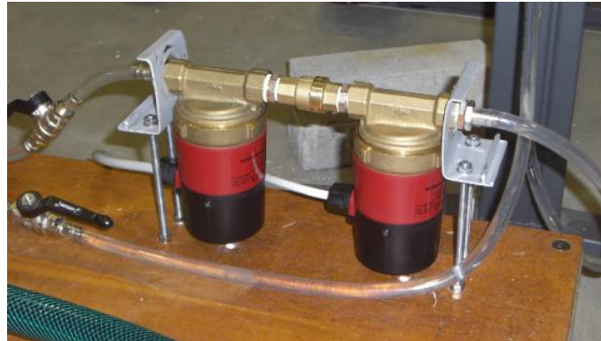
Figure 2.13. Detail of the secondary pumps.
