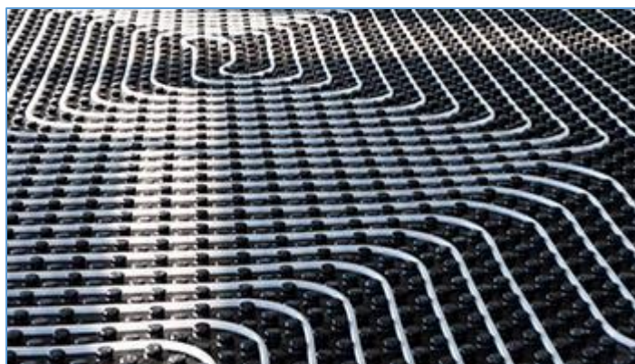
Figure 181 underfloor heating pipes
