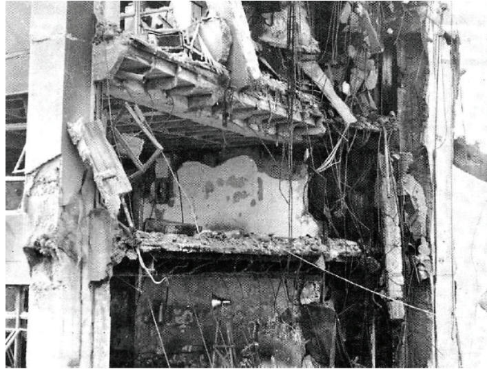
Figure 10: CESP 2 Core Collapse in Sao Paulo, Brazil.
