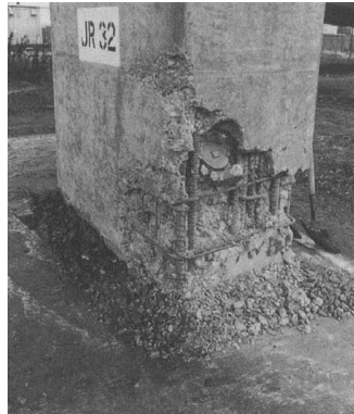
Figure 3 : Lap-splice bond column failure, Loma Prieta bridge 1989
