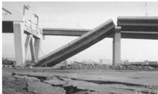
Figure 2 : Nishinomiya-ko bridge following Kobe earthquake, 1995
