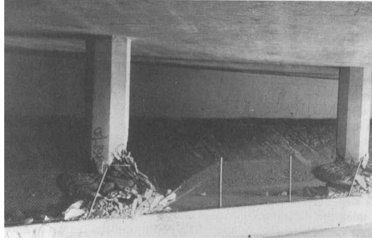
Figure 4 : Bull Creek Canyon Channel Bridge damage in 1994 Northridge earthquake
