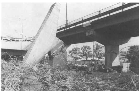
Figure 6 : Flexural-shear failure at pier mid-height of Route 43/2 overpass, 1995 Kobe earthquake
