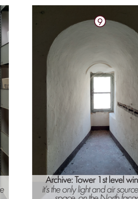
Archive: lower 1st level entrance the stairs obtained in the masonry of the Tower to reach its 1st level
