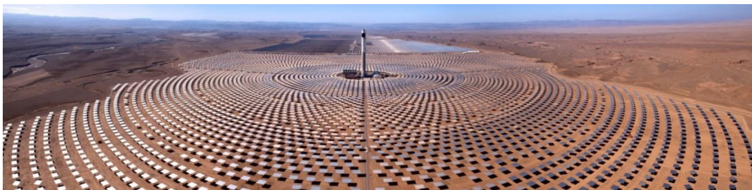
Figure 1-1 Ouarzazate, Morocco, NOOR power plants
