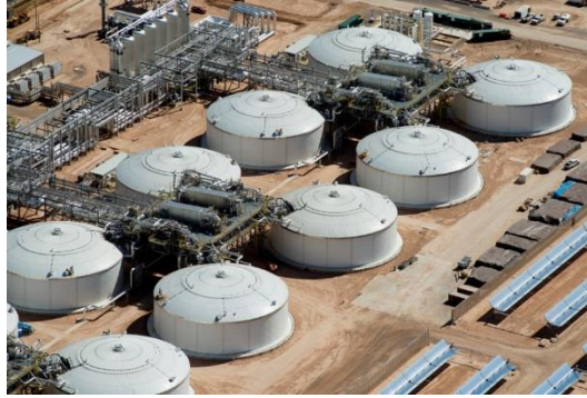
Figure 3-8 Molten salt storage tanks
