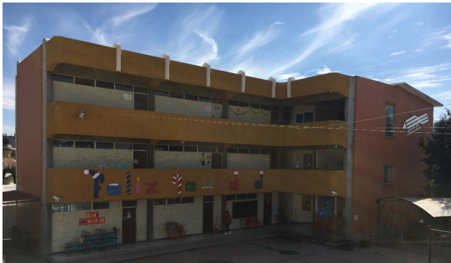
Figure 3.3 Current state, during the inspection done in January 2020 (Source: CEEH photographic register)
