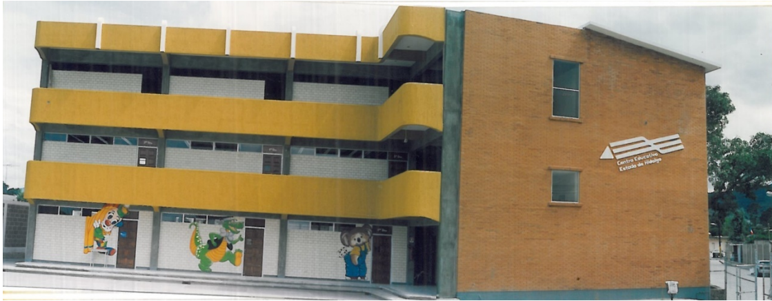
Figure 3.2 As built state, with the main unit finished and the expansions postponed for future growth. (Source: CEEH photographic register)
