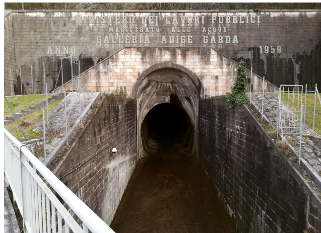
Figure 1.3: Discharge point of the Mori-Torbole tunnel. Picture taken by the author
