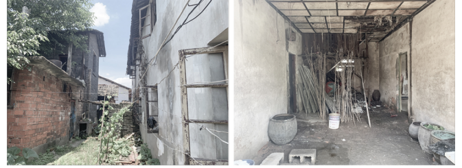
1 | MV: The building was built in the Republic of China period, belonging to the common folk houses MQ: The building can not be used, the structure is unstable
