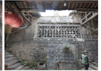
MQ:The structure is stable, the main components are relatively complete, the interior and exterior decoration is dilapidated
