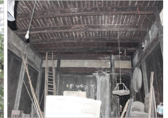
MQ:The building can be used, the structure is stable, the main components are missing and dilapidated
