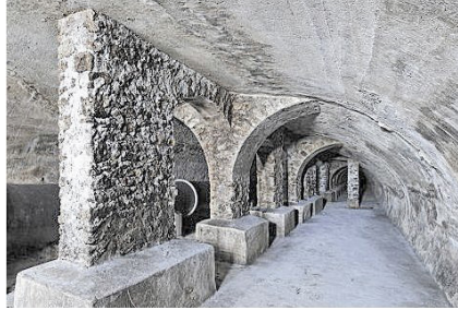
6 Fushougou drainage system
