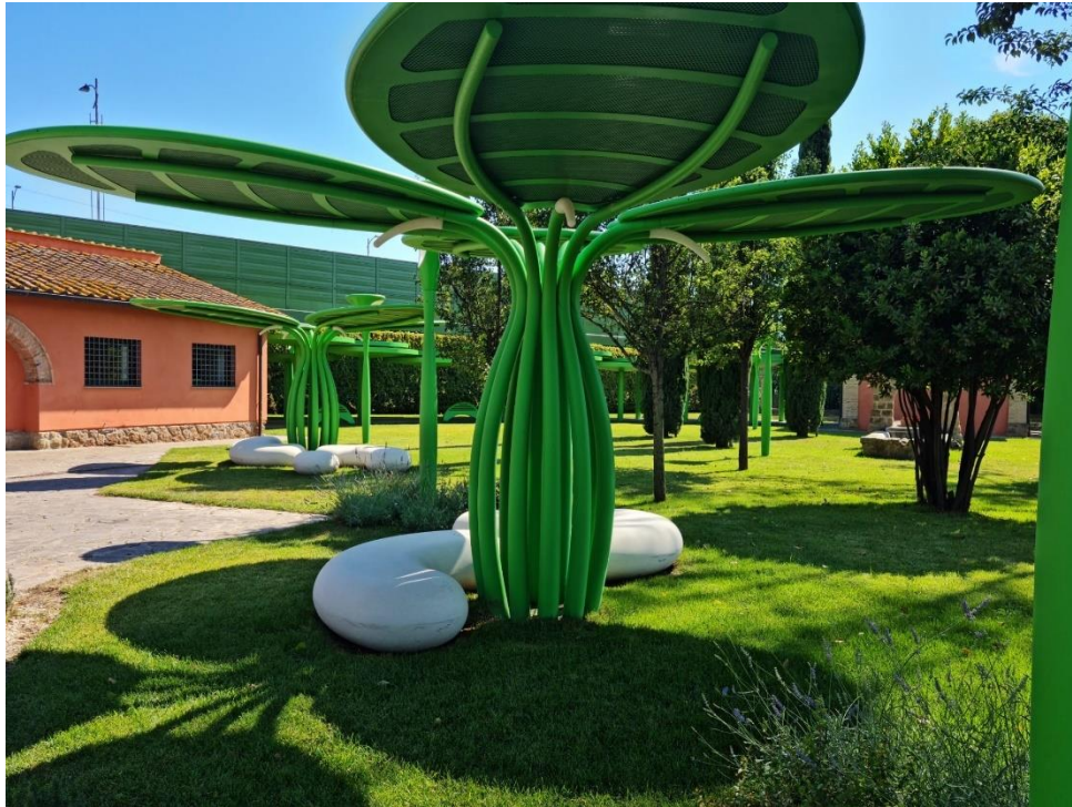
Figure 2. 5: Solar Panel for energy generation in Green Island
