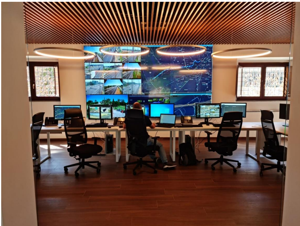
Figure 2. 6: Control room in Green Island
