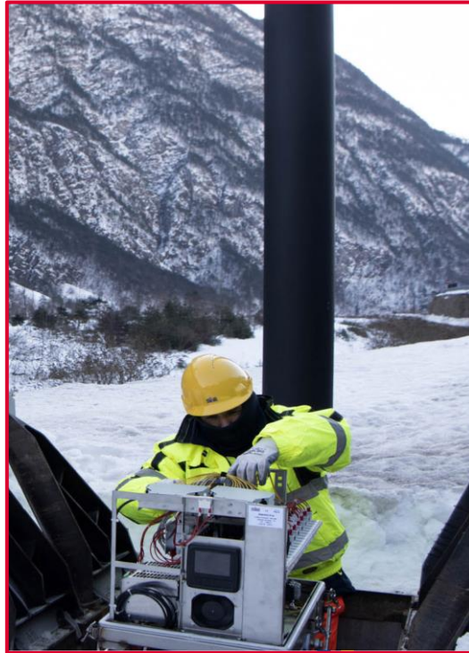
Figure 2. 10: Technology Energy Gate of Roadside Unit
