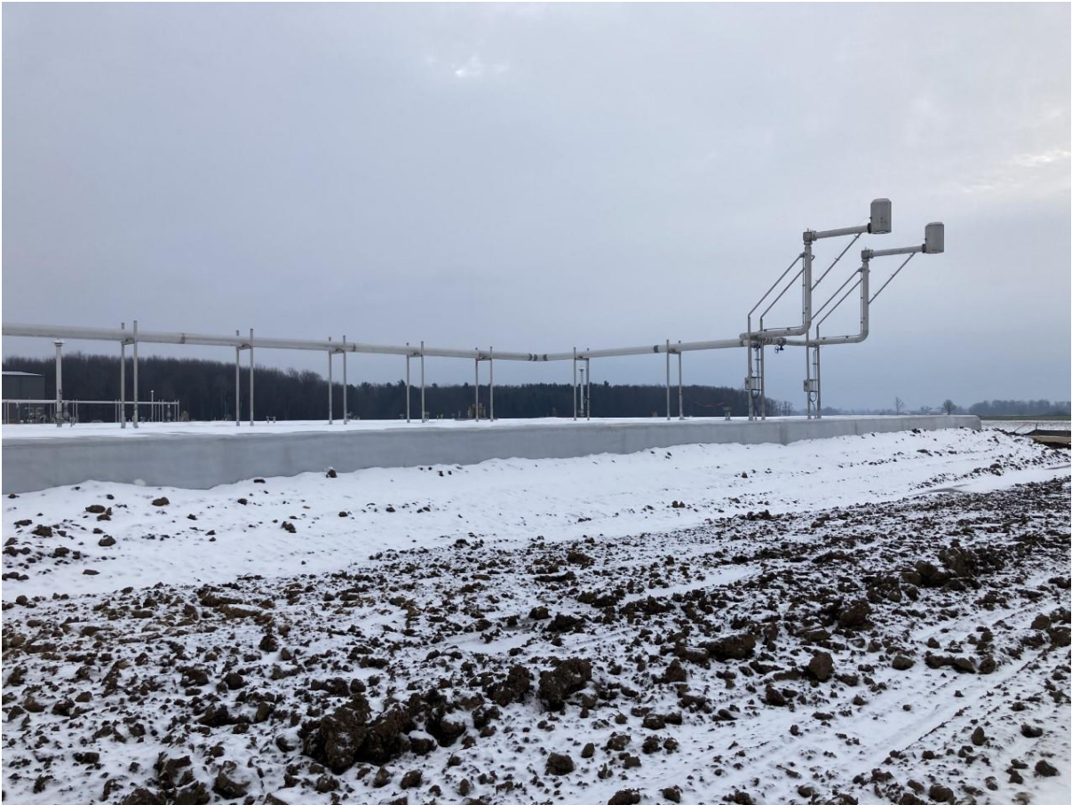
Figure 4.1.9 Flare from plug flow digester in case upgrading facility can not receive raw biogas due to maintenance.
