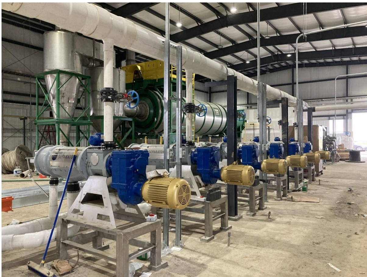
Figure 4.1.12 Solids separation facility for recycled bedding.
