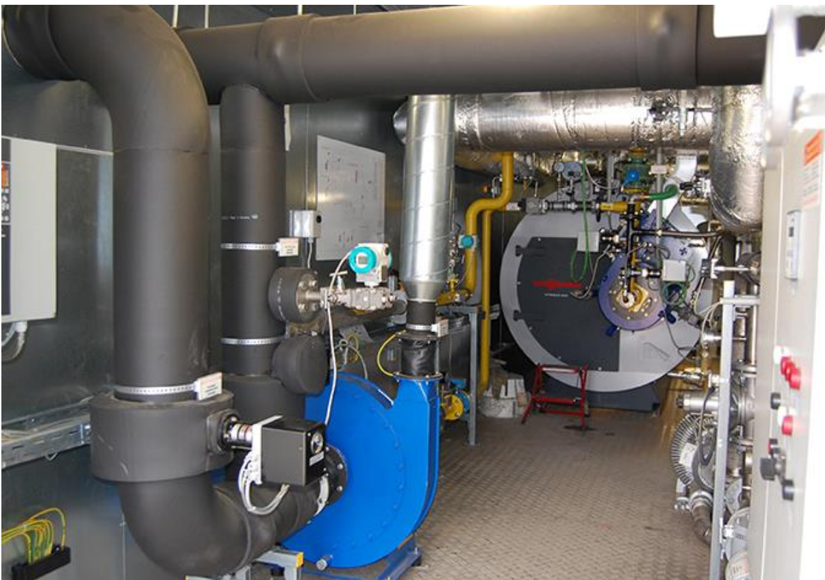
Figure 4.2.3 Mechanical Room of Arneburg Biomethane Refinery
