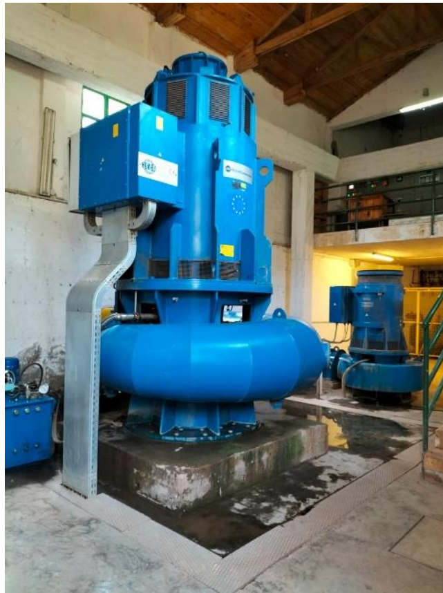
Figure 1.5: Turbines in the Ikondo hydropower plant.
