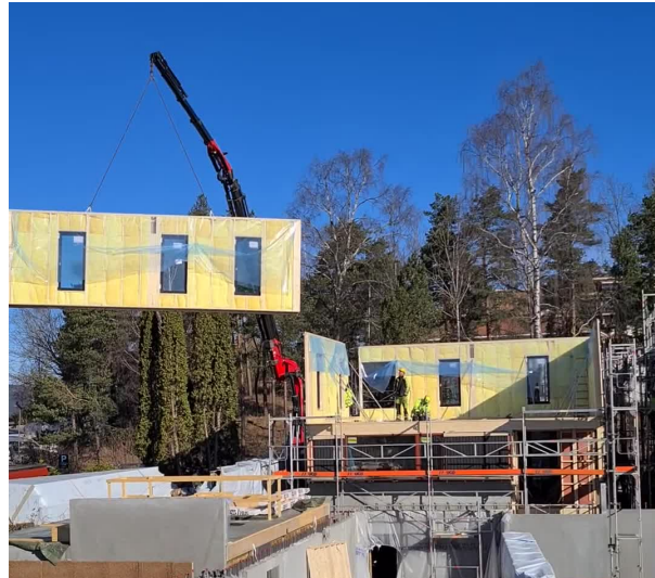
Figure 1.1: Example of installation of a wall element in a construction site in Oslo, Norway. Source: author personal collection.
