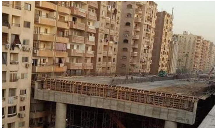
Figure 18 Example for Wrong Bridges Planning
