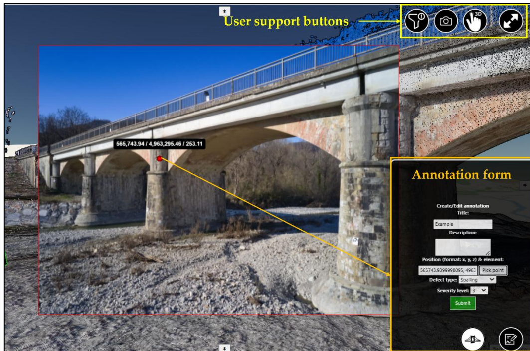
Figure 47. The interface allows users to inspect a textured 3D model of the bridge and record defect annotations by selecting a point directly on the geometry. Each annotation captures spatial coordinates, defect type (e.g., spalling), severity level, and optional textual descriptions. This integration facilitates consistent documentation and streamlined condition assessment in a spatially aware environment (from Gaspari et al., 2025b).
