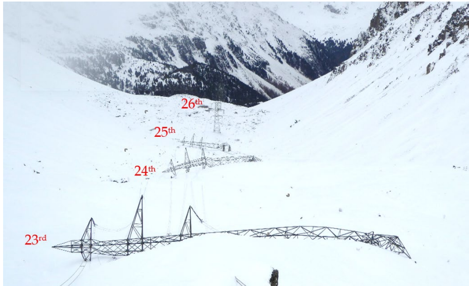
Figure 0.1: Towers from n23 to n26 after the storm in 2018 (source SwissGrid ).
