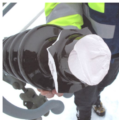
(b) Broken insulator in tower n22.
