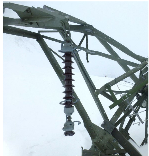
Figure 6.10: Broken insulator, tower n22, position 32, the closest to the limit (Figure 6.8).
