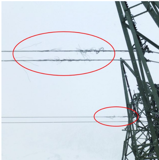
Figure 6.9: Damaged cable in tower n22, positions 12 (back) and n22 (front), which were close to limit load (Figure 6.7).
