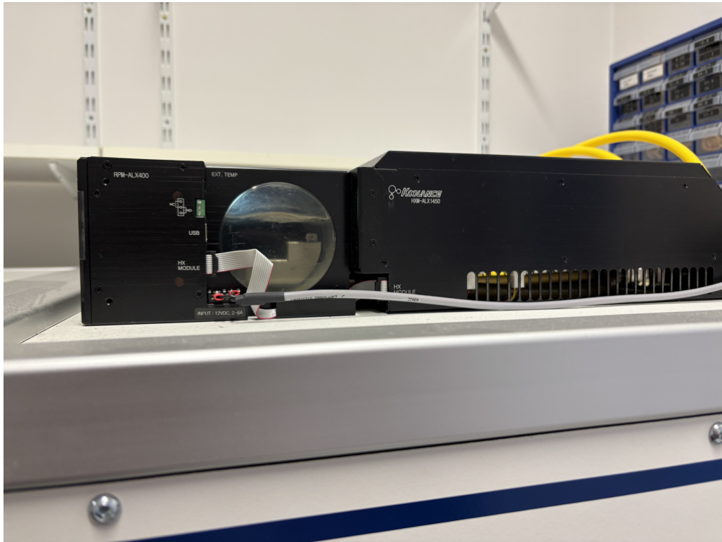
Figure A.4: Cooling system of the CORALIS system.
