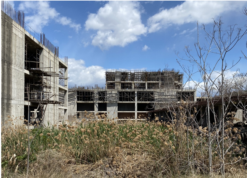
Figure.8 Title: Wild flora in the level foundations of the VOVOS' Shopping Mall, 2021 Source: Author
