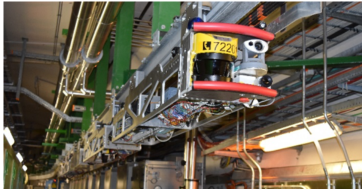
Figure 2.1: TIM robot: autonomous robotic system operating on a ceiling-mounted monorail in the LHC tunnel (27 km long Large hadron collider), composed by different wagons (modular), enabling remote inspections, radiation monitoring, and intervention during beam stops and shutdowns. (Retrieved from [8]).
