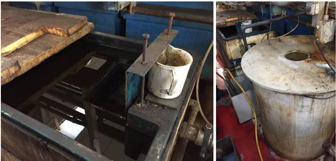
Figure 15 - Oil separator (on the left) and its recovery tank (on the right)
