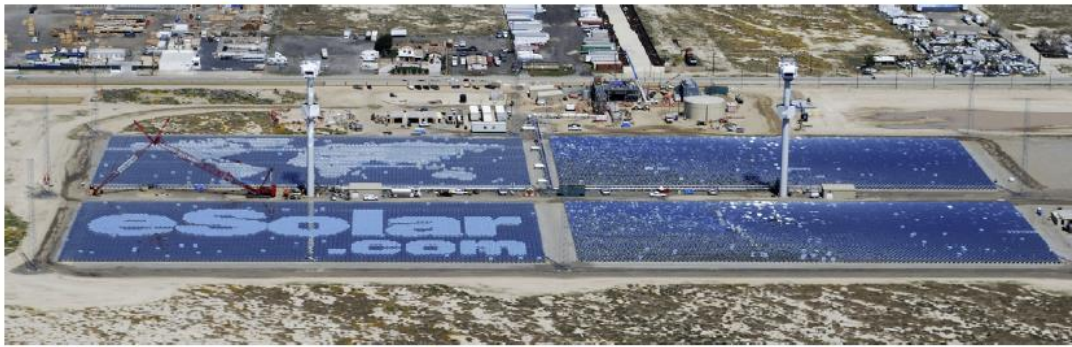
Figure 22 Sierra SunTower Facility
