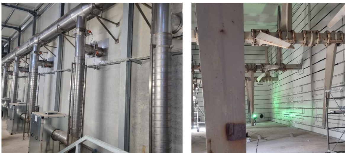
Figure 17: internal view of the PFR digester with the heating system pipes (left) and the mixing system agitator's shaft and blades (right).
