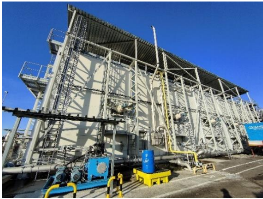
Figure 15: PFR digester external view.
