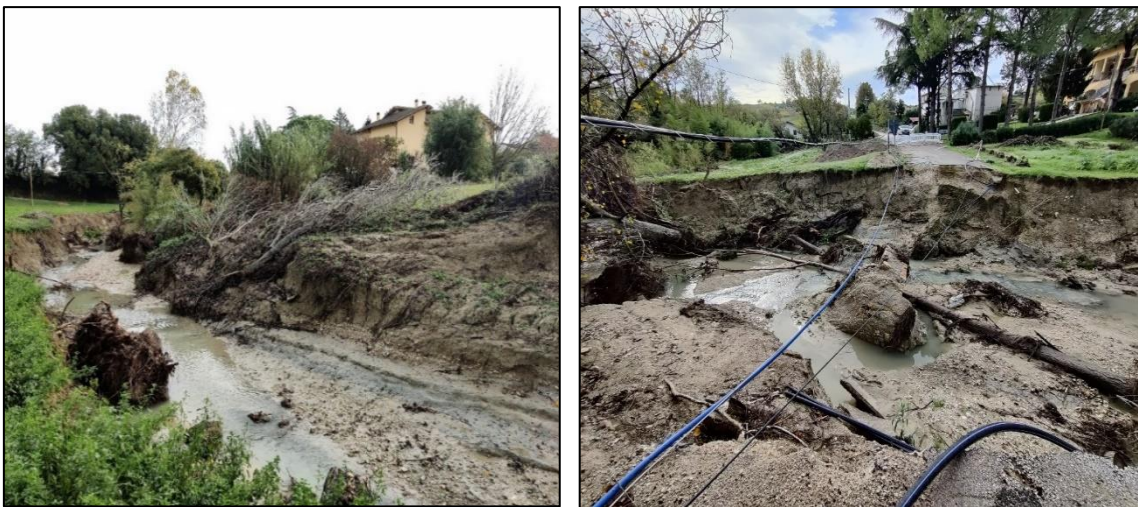
Figure 4: a), b) Examples of bank erosion along Misa stream.
