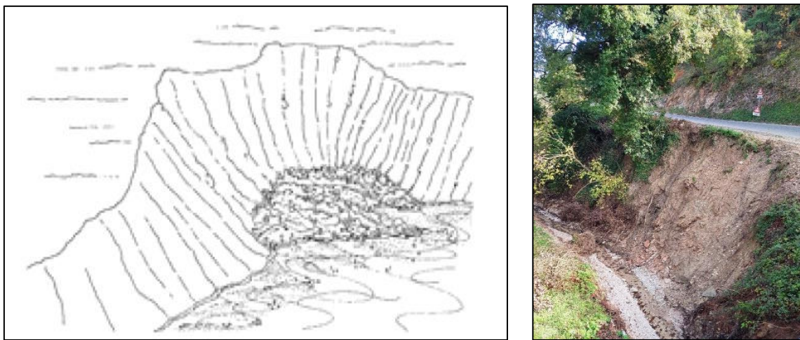
Figure 6: a) Mass failure (36); b) Mass failure along Misa stream.
