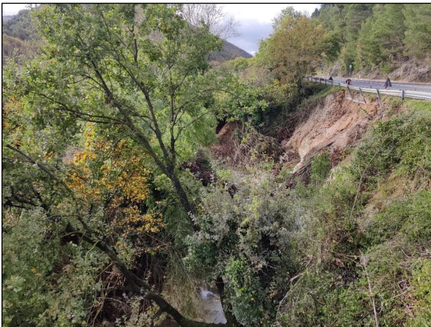
Figure 7: Shallow landslide in the municipality of Arcevia.
