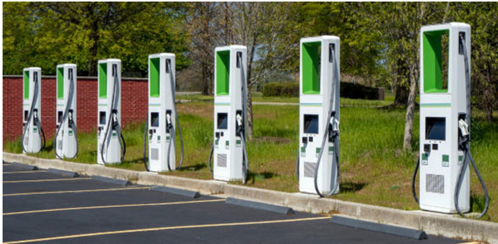
Figure 1.7: Charging station with 7 Mode 4 EVSEs.
