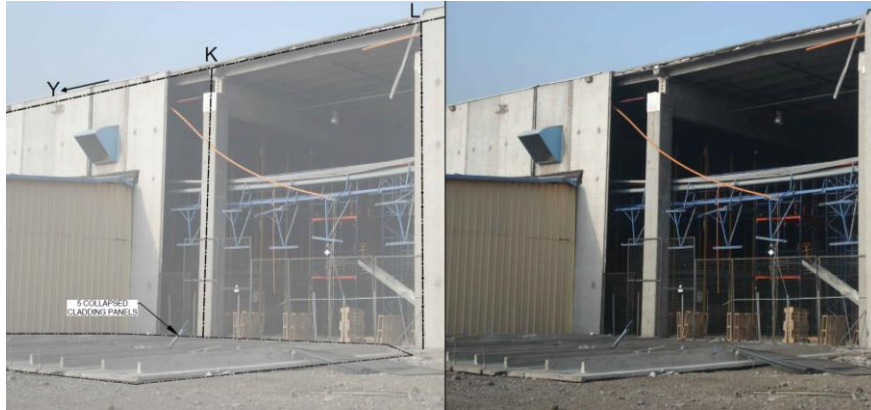
Figure 4-4: Overturning of cladding panels in direction Y
