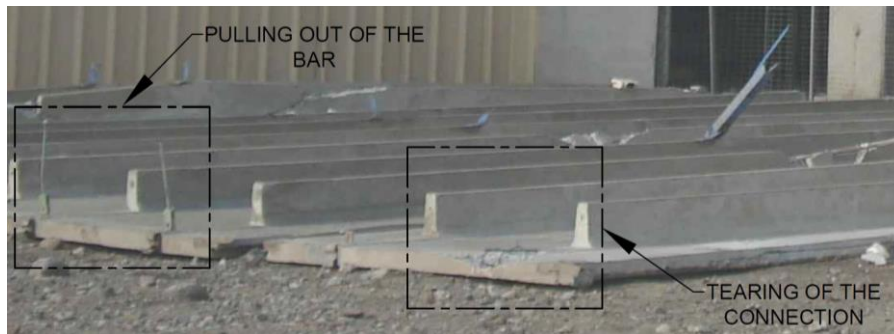
Figure 4-5: Indication of the mechanism of failure on the cladding panel connection.
