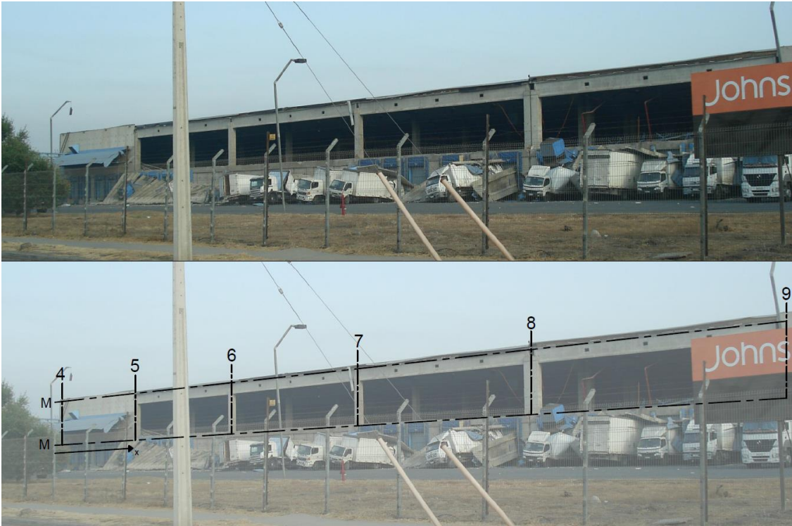
Figure 4-3: Cladding panels collapsed in axis M picture 2.
