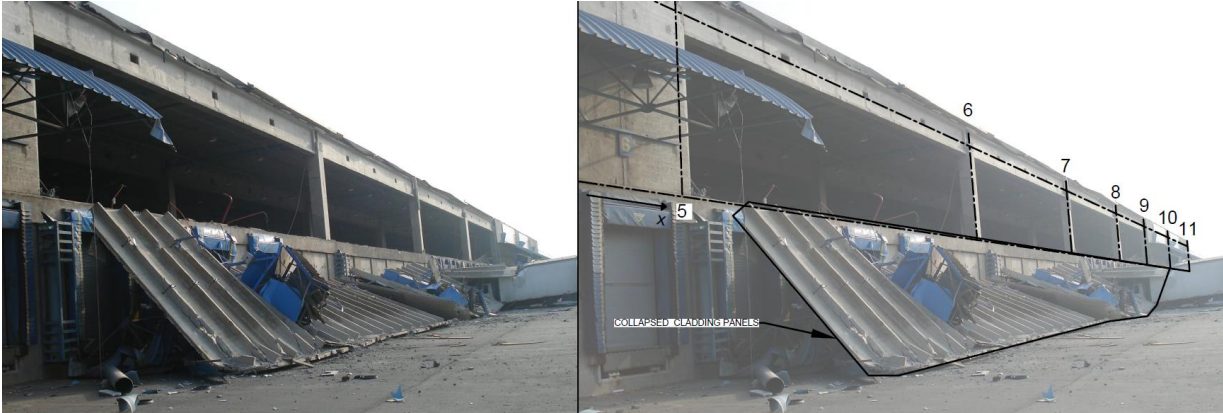
Figure 4-2: Cladding panels collapsed in axis M picture 1.
