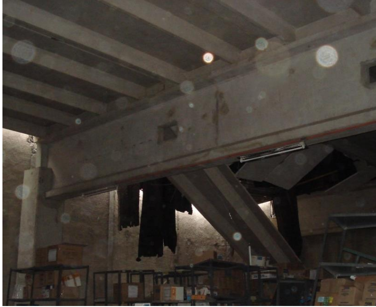
Figure 4-9: Collapsed of one roof slab.
