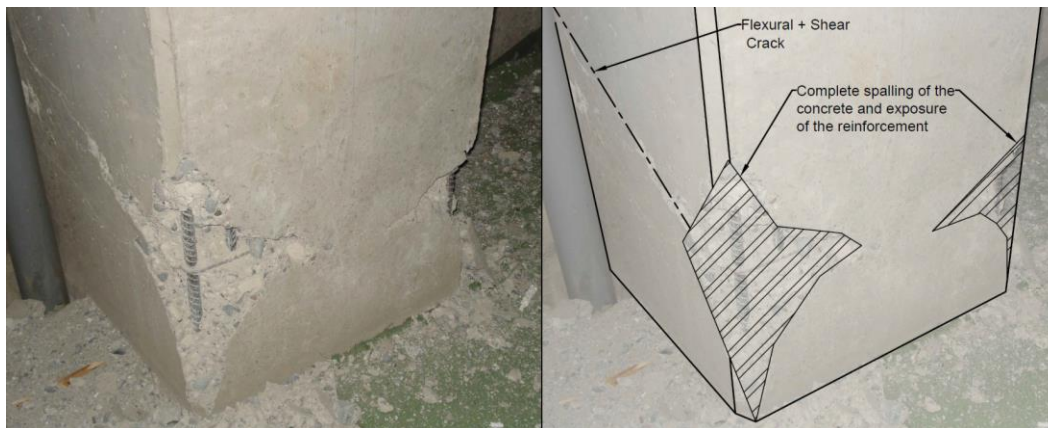
Figure 4-6: Detail of damage at the columns' base.
