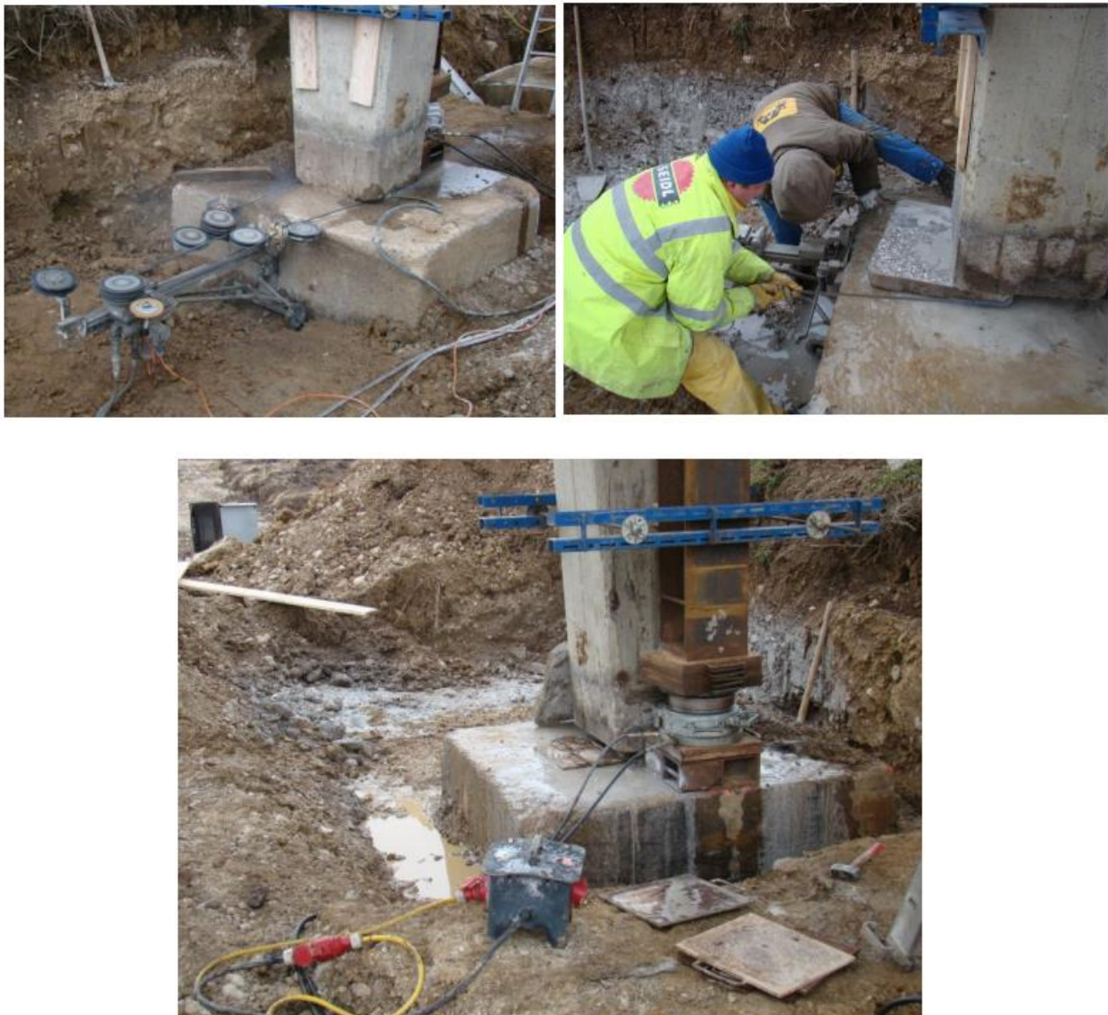
Figure 6 - a) Cutting of the pier; b) insertion of the steel plates; c) lowering with a hydraulic jack
