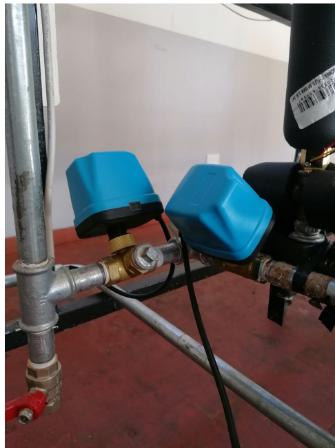
Figure 4.6: Valves. Specifically in the photo are shown the two valves that handle the bypass of the secondary circuit.
