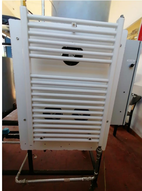
Figure 4.10: Secondary Heat Exchanger. From the picture, it can be seen the three fans mounted behind the component for additional flow cooling.
