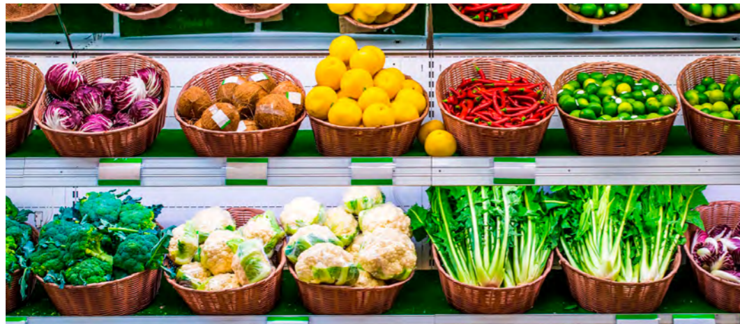
Fig.63 Refrigerated storage of fresh produce at grocery store.
