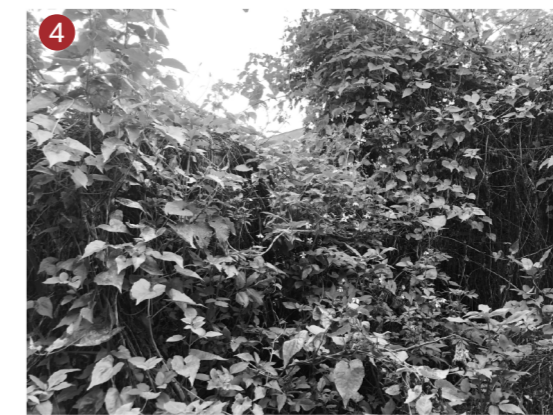
Plants have flooded the building, affecting building lighting.
