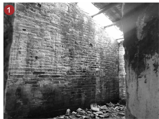
Part of the roof collapsed, with tiles strewn across the ground
