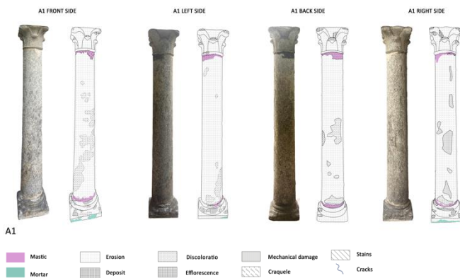
Figure 34: Material and decay mapping on a column of Chiostro della Memoria east façade
