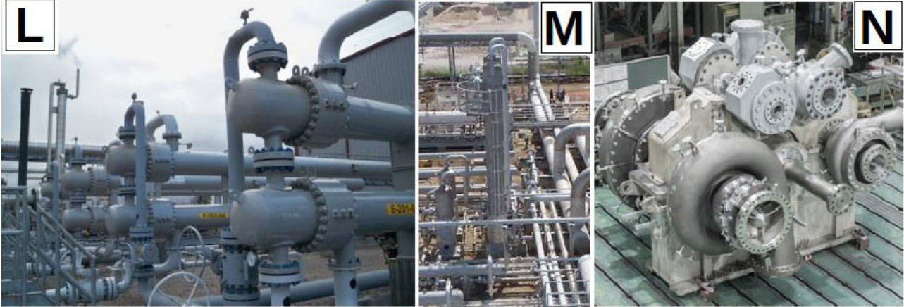
Figure L: representation of the CO 2 interstage heat exchangers in an existing CO 2 compression facility (Coffeyville). Figure M: TEG drying column in an existing CO 2 compression facility. Figure N: integrally geared CO 2 compressor (MHI)
