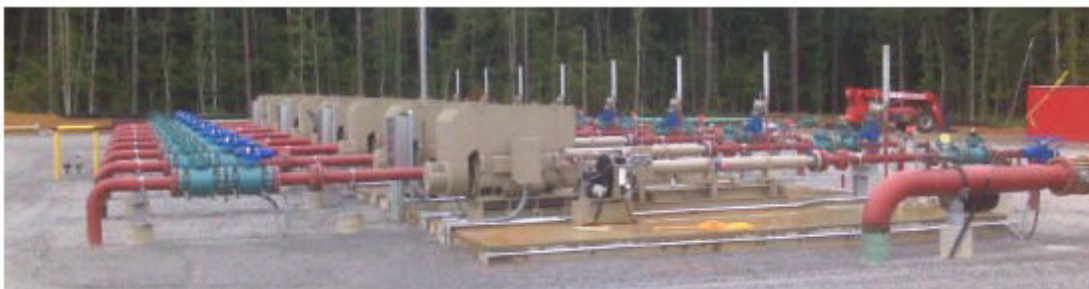
Figure P: carbon dioxide boosting station
