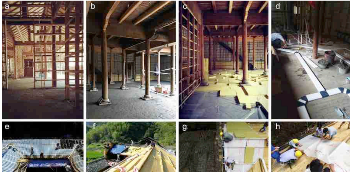
Figure 2-20 Photos during construction of the Aoni No. 3 Courtyard House project, a: replacement and addition of wooden building elements; b: pouring terrazzo floor; c: floor insulation; d: fresh air system channel; e: laying of roof tiles; f: roof insulation (rock wool) and breathability film. g,h: laying of roof vapor barrier film; Source: HXP Planung GmbH.
