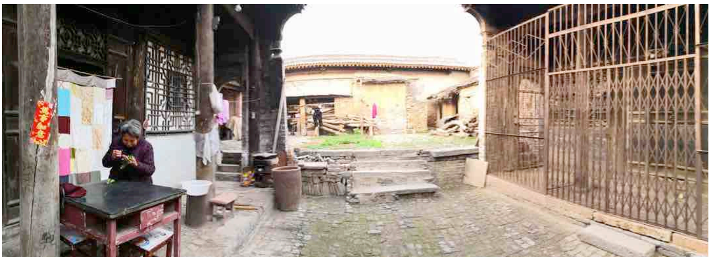
Figure 3-31 The main building in a traditional courtyard was demolished for sale. Photographed by the author in Qing-Shui Village in March 2018.
