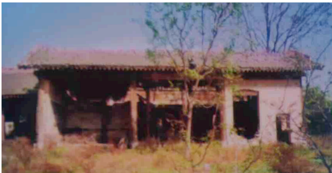
Figure 3-40 The Xian Dian of Guan Yu Temple in Zhang Dai Village in 2000 (before collapse). Source: The Genealogy of the Zhang Dai Village .
