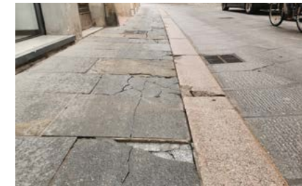
The sidewalk is ruined due to the transit of cars and trucks
