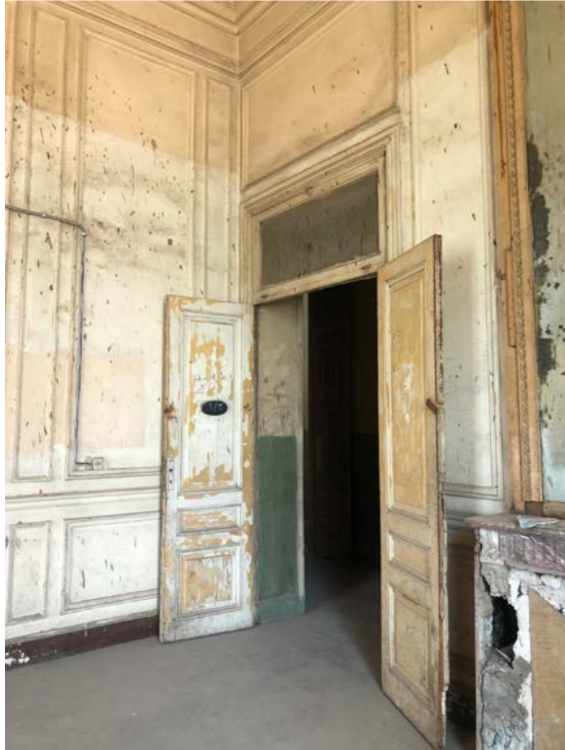
Damages to the Walls and Doors
