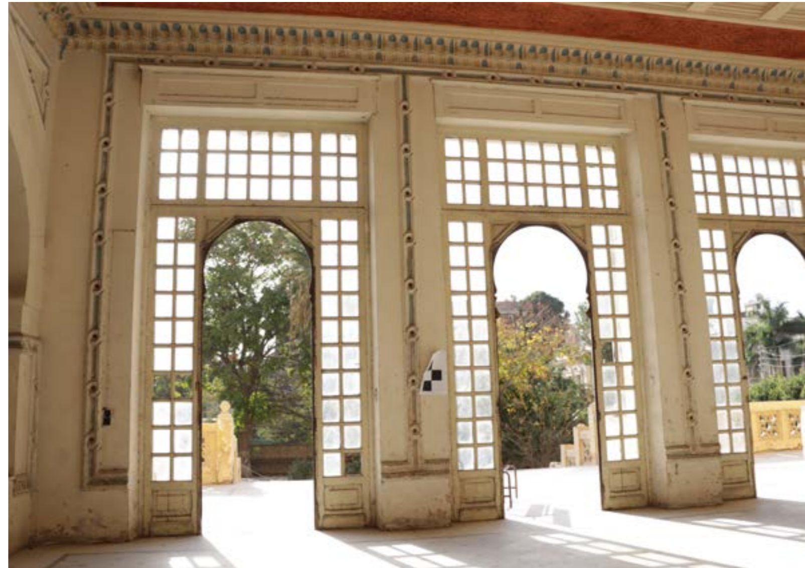
Inconsistent Painting of the Ornaments and the Ceiling
