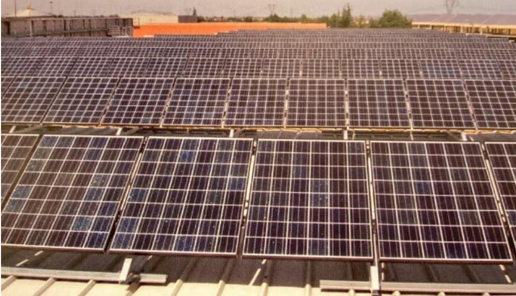
Figure 1.8: PV modules in a 49.7 kWp installation on a rooftop [13].
